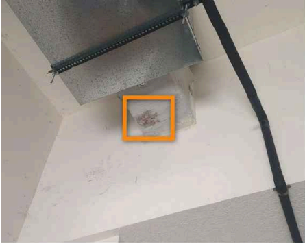
Mold - Air Handler Duct
