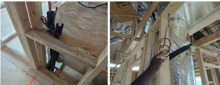
Thermostat wire upstairs hallway
